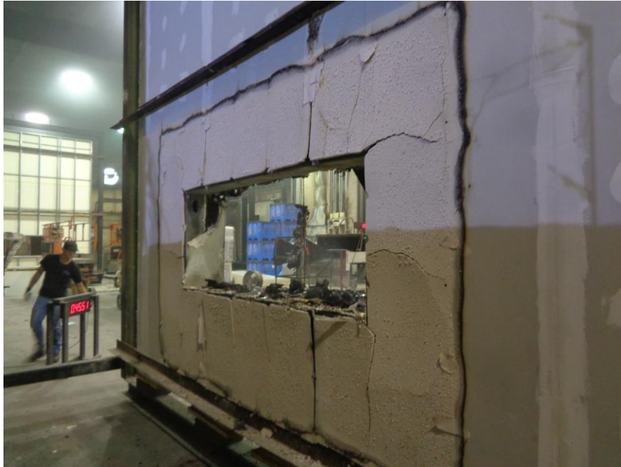
Photo No. 13 Interior First and Second Story Burn Pattern (Post-test)
